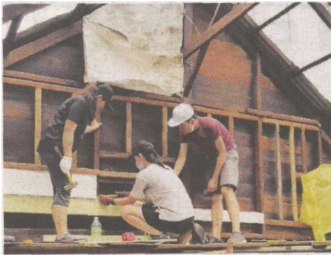
UCSI University and Chung Yuan Christian University architecture students working together to build a communal centre.
